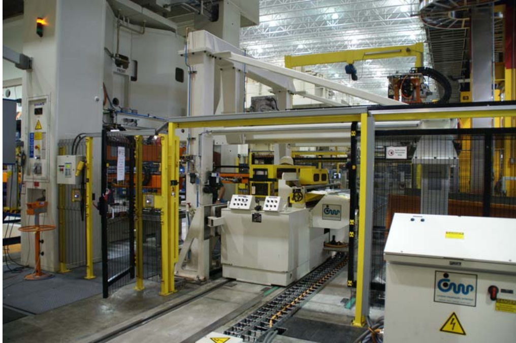
CWP feed unit rail mounted and integrated with Schuler's Destack and Transfer System. Note the feed control HMI mounted on the security fence adjacent to the press column
